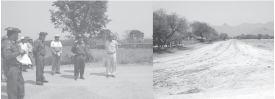
Lt-Gen Ye Myint inspects progress in construction of No 2 Thazi-Hlaingtat-Tatkon road. — MNA
