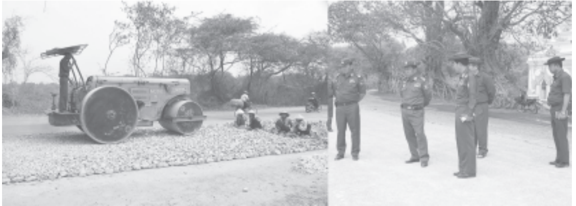
Lt-Gen Ye Myint inspects laying of gravel on Taungthaman Lake ring road.—MNA
