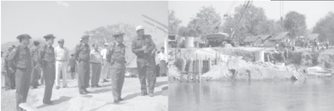
Lt-Gen Ye Myint oversees construction of Naungkham Bridge (Thanywa) crossing Zawgyi River. — MNA
