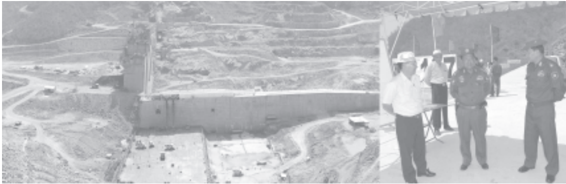
Lt-Gen Ye Myint inspects progress in construction of Yeywa hydel power project.
