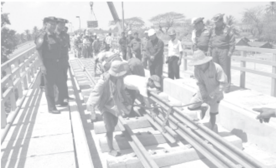
Lt-Gen Maung Bo oversees progress in laying rail tracks on Mottama side. — MNA
