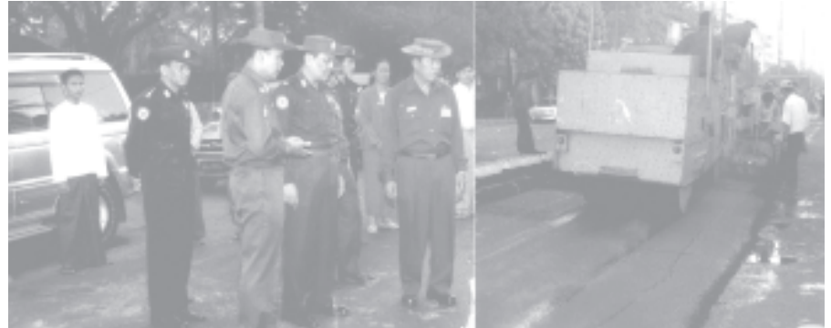
Commander Brig-Gen Hla Htay Win and Mayor Brig-Gen Aung Thein Lin inspect tarmacking on U Chit Maung Road in Bahan Township. — MNA
