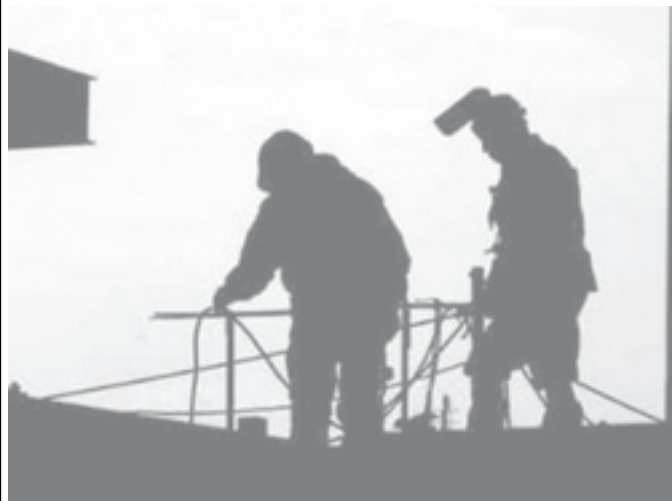
South Koreans work at a construction site in Seoul, on 16 Feb, 2006. —INTERNET
