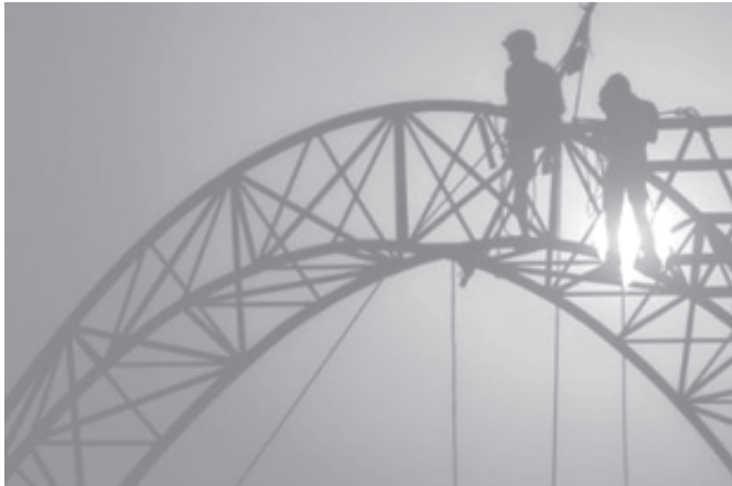
Indian construction workers build a toll plaza on the national highway at Sankrail village, about 30 km (19 miles) southeast from the eastern Indian city of Kolkata, on 15 Feb, 2006. —INTERNET
