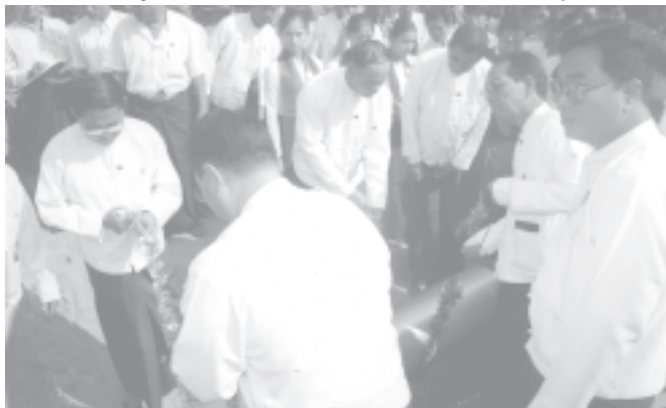
Mayor Brig-Gen Aung Thein Lin, Vice-Mayor Col Maung Pa and officials laying water pipeline to supply water to Waibargi Myothit, North Okkalapa Township. — YCDC
