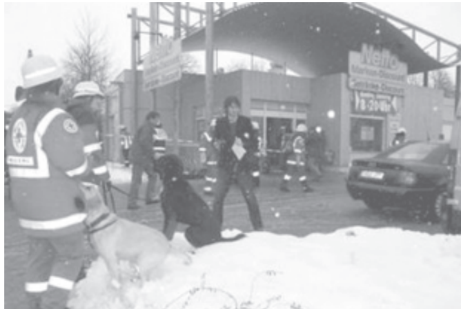
Emergency services attend the scene of a damaged supermarket in Toegling am Inn, east of Munich on 7 Feb, 2006. The flat roof of the Netto Sued supermarket in southern Germany gradually collapsed amid heavy snow on Tuesday.—INTERNET
