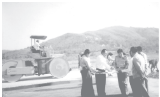
Deputy Minister for Transport Col Nyan Tun Aung inspects extended construction of runway of Mawlamyine Airport. — MNA
