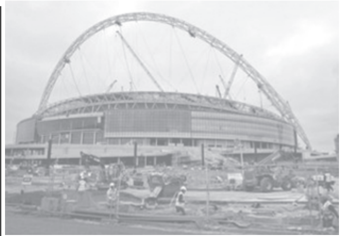
A general view shows building work continuing at the new Wembley Stadium in London, on 30 Jan, 2006. The new Wembley Stadium has a 70 percent chance of being ready for the FA Cup final in May, project officials said on Monday. —INTERNET
