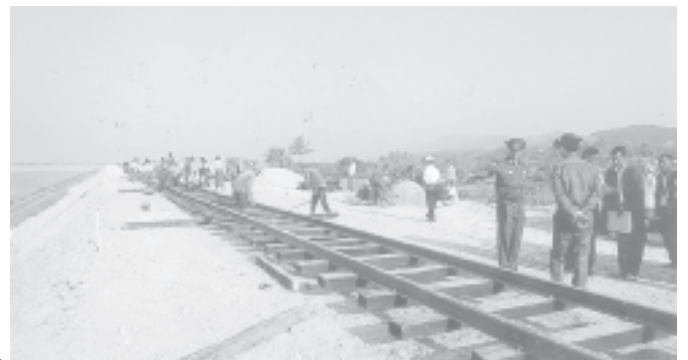
Minister Maj-Gen Aung Min inspects laying of sleepers on the bank of Mottama. — RAILWAYS
