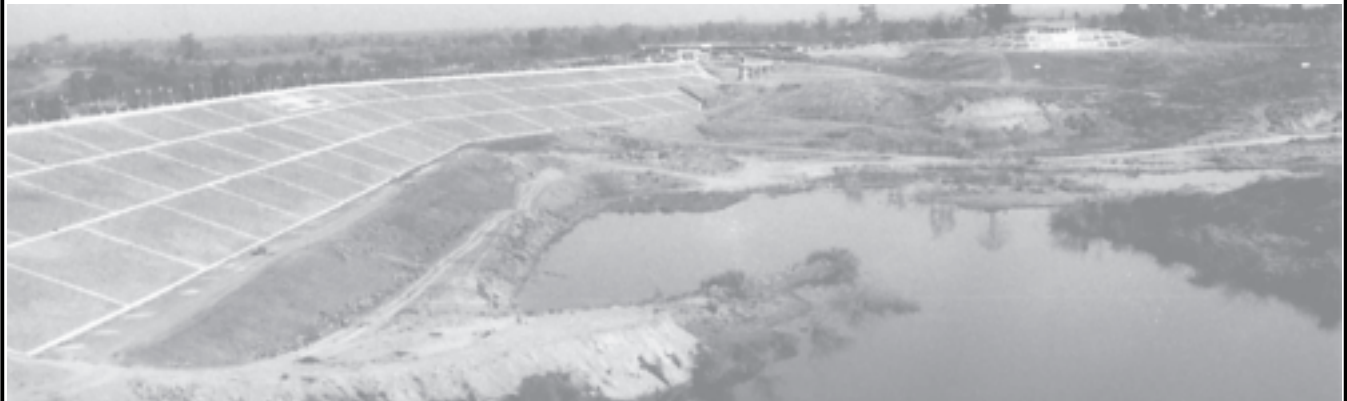
Completion of Pade Dam built by Construction-3 of the Irrigation Department near Shwepandaw Village of Aunglan Township on 16-1-2005. The dam is an earthen one measuring 118 feet high and 2,400 feet long situated in Pade Creek, 36 miles from Aunglan.
