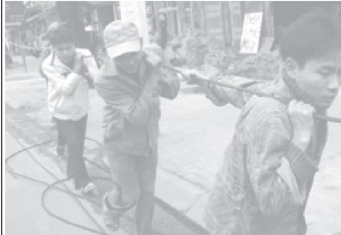
Vietnamese workers pull a telephone wire to set up new telephone lines in Hanoi on 20 Jan, 2006. —INTERNET
