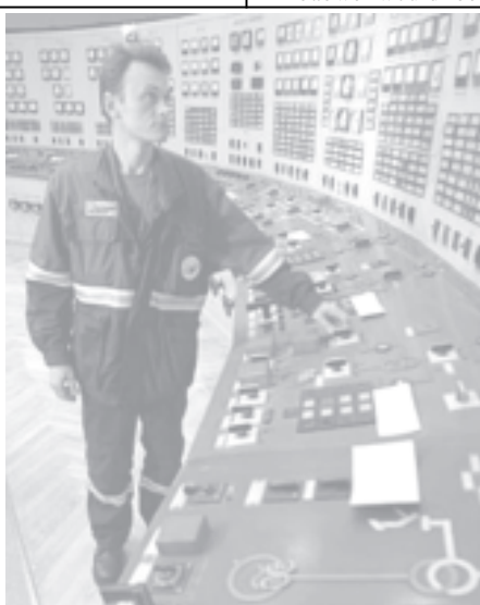
An operator presses a button in the control centre of a central heating station in southwest Moscow on 20 Jan, 2006. This station produces hot water for heating and electricity for southwest Moscow.
