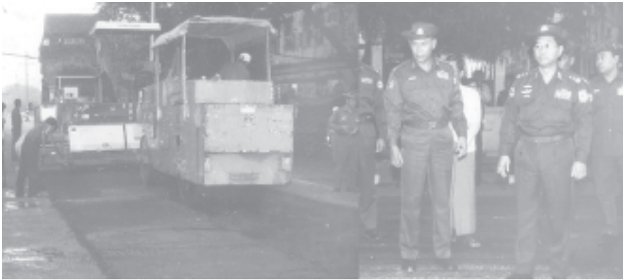
Commander Lt-Gen Myint Swe and Mayor Brig-Gen Aung Thein Lin inspect repaving of Bogyoke Aung San Street. — MNA
