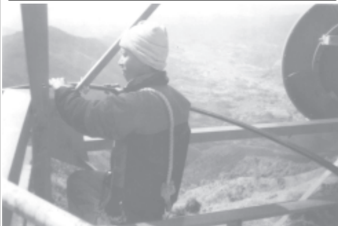
Cables being put into service at microwave station in Salangyi Township, Monywa District, Sagaing Division.
