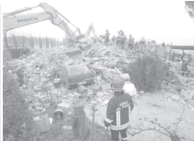
Firefighters and rescuers search through the rubble of a collapsed building destroyed by a gas explosion, in Quarrata near Pistoia, Italy, on 29 Dec, 2005. Two people died in the explosion police said.—INTERNET
