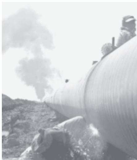
Iraqi workers repair a pipeline as smoke from a fire billows in the background on 15 Dec 2004.—INTERNET
