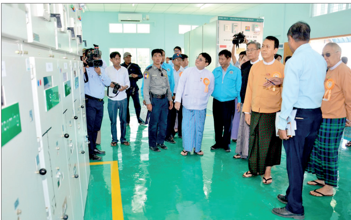
Two 33/11 kV, 5 MVA power sub-stations inaugurated in succession. PHOTO:MOEE
