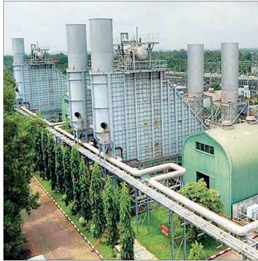
Thakayta gas fired power station in Thakayta Township
