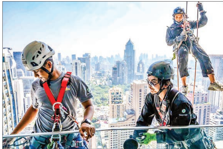
Workers scale a skyscraper to install Christmas and New Year lights in Bangkok on 10 December, 2019. PHOTO: AFP
