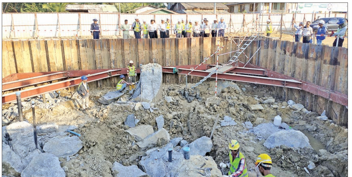
Union Minister U Han Zaw inspects the construction site of the project area of the Korea-Myanmar Friendship Dala Bridge yesterday. PHOTO: MNA
