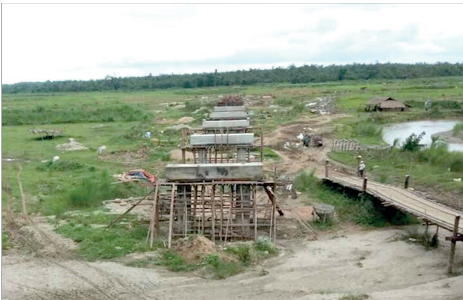
Construction work of Pyaungthwe Bridge in Kyunhla Township, Sagaing Region is 35 per cent finished. PHOTO: IPRD
