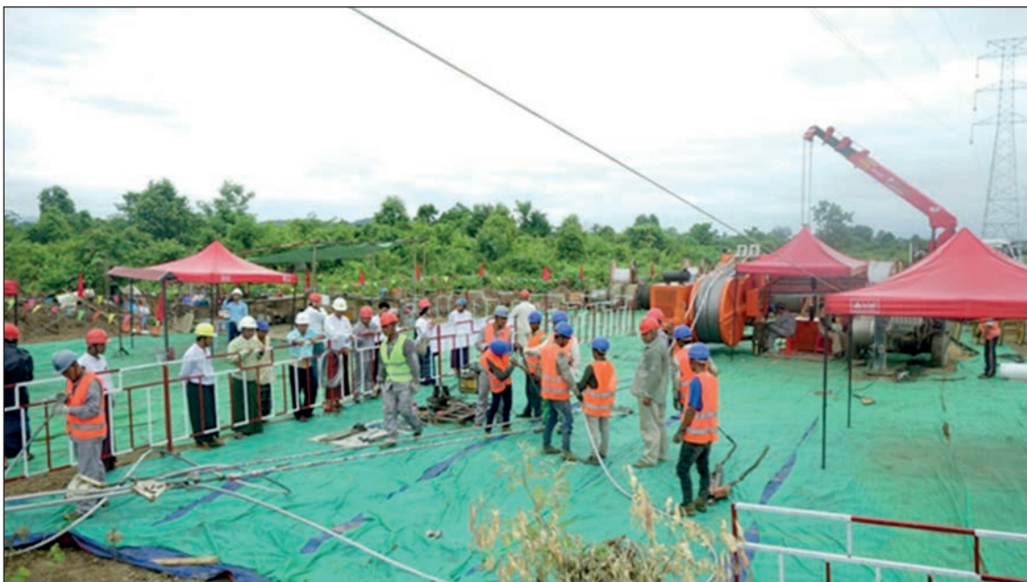
A 230 kV power transmission line is designed to distribute electricity generated by Tarpein-1 Hydropower Plant to households in ten townships in Sagaing Region. PHOTO: IPRD
