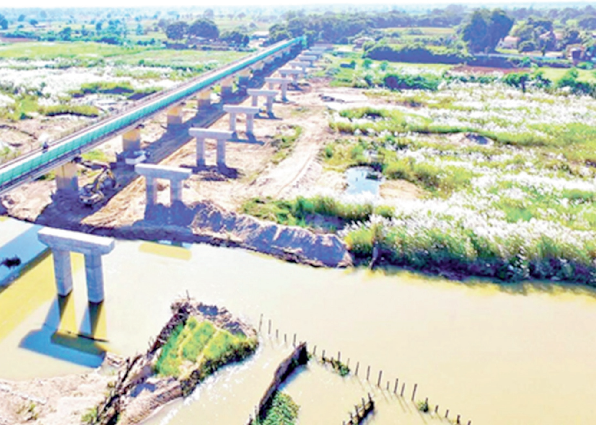
A new bridge in parallel with the Mu River crossing bridge in Sagaing Region is being built by Ministry of Construction. PHOTO: IPRD
