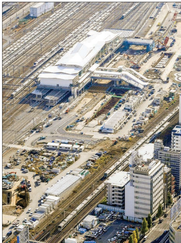
Photo taken on 14 November 2019, from a Kyodo News helicopter shows Takanawa Gateway Station in Tokyo, East Japan Railway Co.'s new Yamanote loop line station under construction. PHOTO: KYODO NEWS
