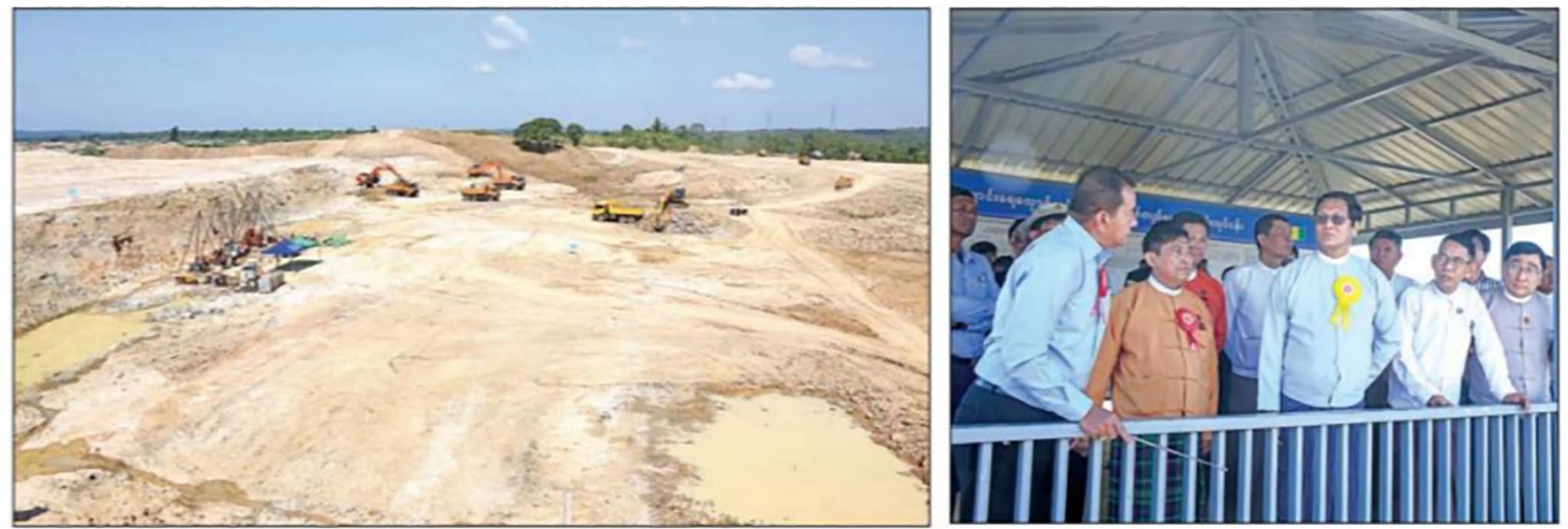
Vice President U Henry Van Thio inspects the construction of new spillway of the Swa Chaung Dam in Yedashe Township yesterday. PHOTO: MNA
