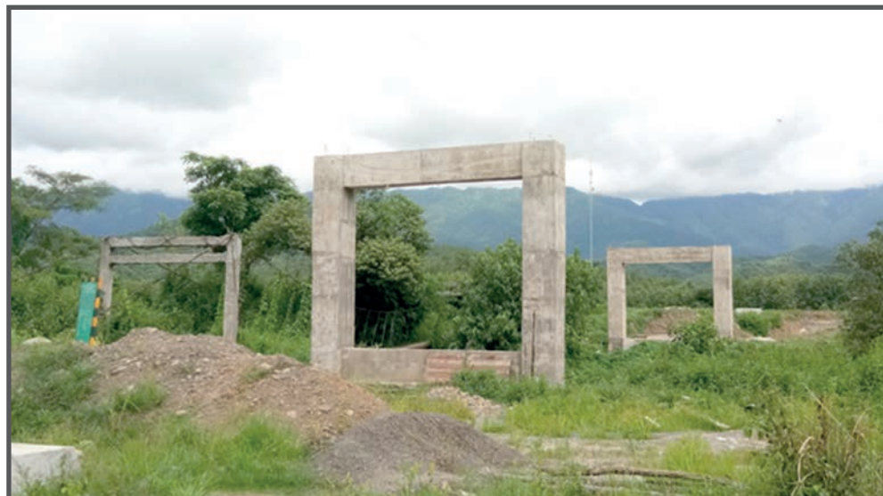
A rural suspension bridge is being built in Kyeekha Town, Chin State. PHOTO: IPRD
