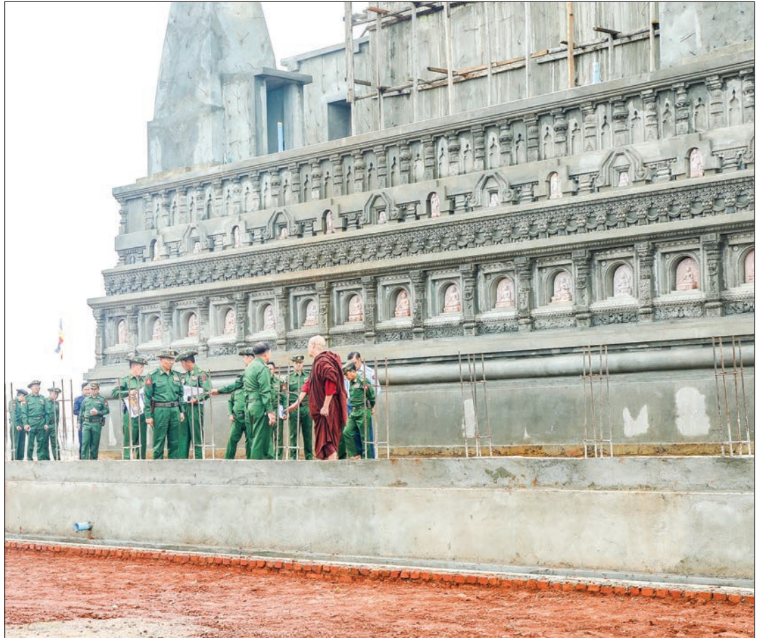
Senior General Min Aung Hlaing and party visit to the Thatta Thattaha Maha Bohdi Pagoda under construction in Buddha Garden compound near Pan Kwe Village in Shan State on 18 October.
