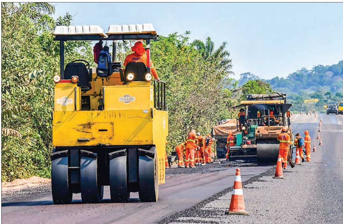
Workers pave the BR163 highway in Itaituba — President Jair Bolsonaro's government is eager to develop the Amazon to bolster Brazil's weak economy. PHOTO: AFP
