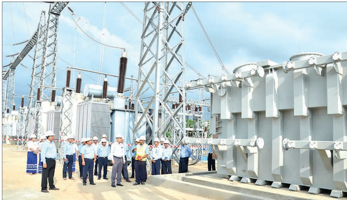
Deputy Minister Dr Tun Naing visits the 230KV Shwesaryan main sub-power station in Patheingyi Township on 5 October. PHOTO: MNA
