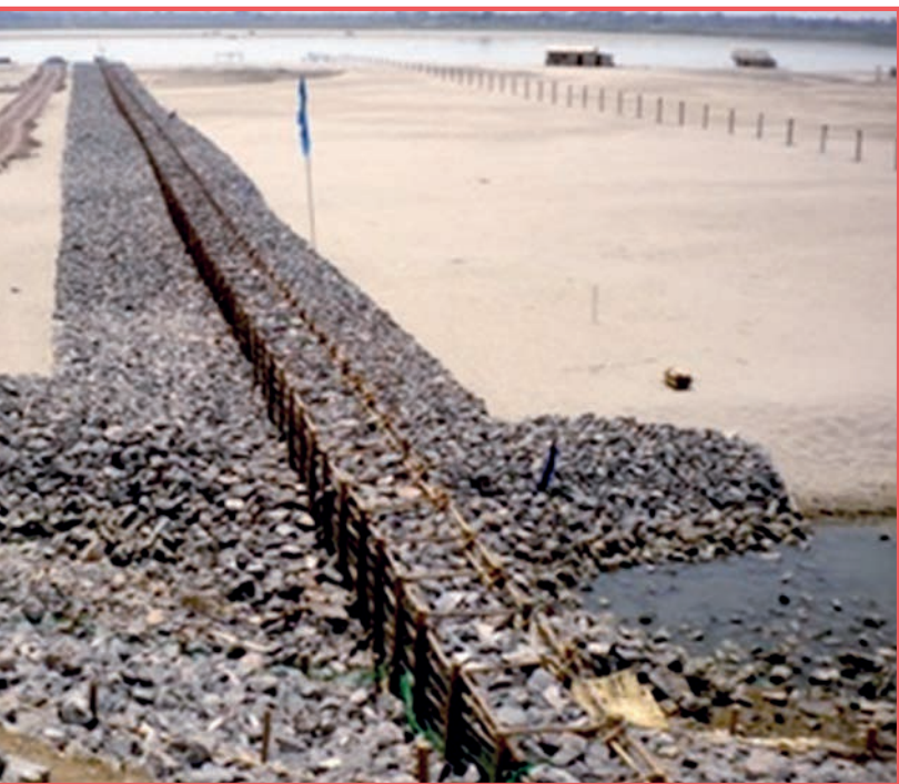
Ks. 5.3 billion would be spent to construct retaining walls in Mandalay Region to solve problem with the riverbank erosion along the Ayeyawady River. PHOTO: DWIR
