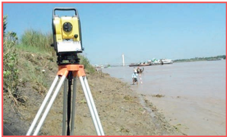
An initial survey on construction of the riverbank protection tasks along the Ayeyawady River in Mandalay Region will be conducted by DWIR. PHOTO: DWIR
