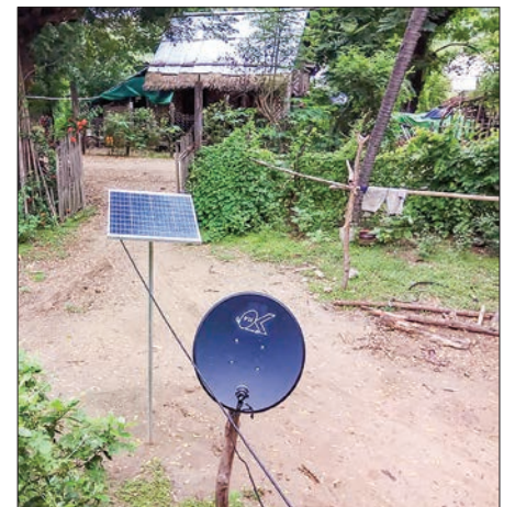
Solar power system installed at a village in Pakokku Township, Magway Region. PHOTO: THAN LWIN
