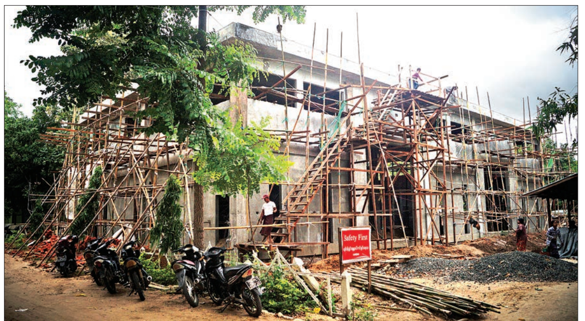
The construction site of regional agricultural machinery workshop in Kanbalu Township, Sagaing Region. PHOTO: AUNG WIN NYEIN (KANBALU)
