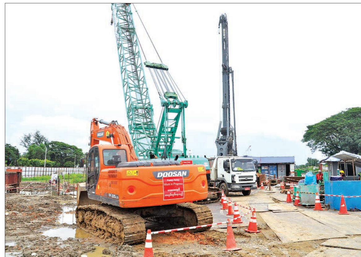
Bored piling machine in operation at the construction site of the new bridge linking Thanlyin and Thakayta. PHOTO: THAN SOE
