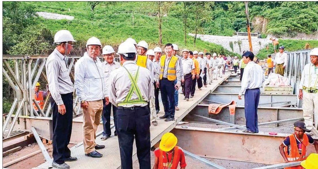
Deputy Minister U Kyaw Linn inspects the construction of Bailey bridge to replace the damaged Gote Twin bridge on 18 August. PHOTO: MNA
