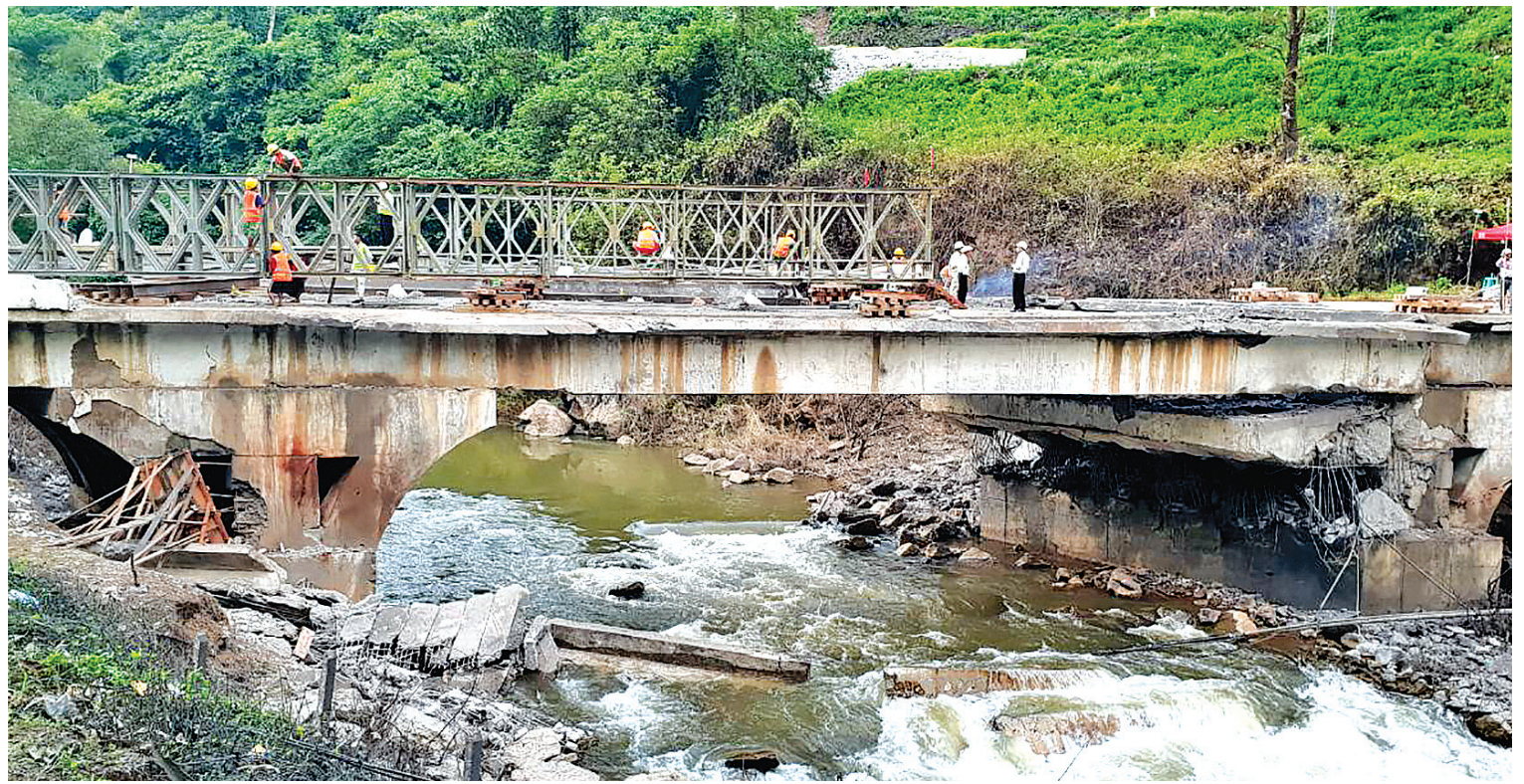
The Special Bridge Construction Teams are building a 210 ft-long bailey bridge to replace the Gote Twin Bridge in Nawngkhio. PHOTO: MNA
