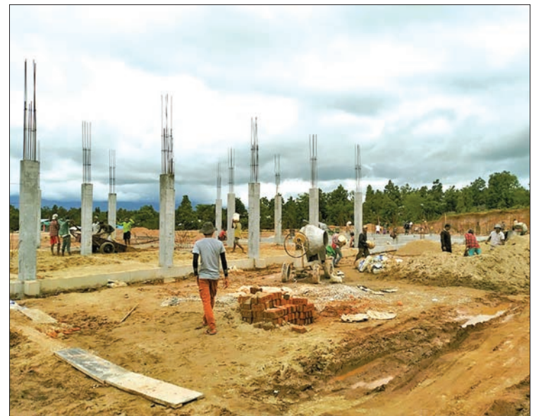
Builder workers work at the construction site of Myanmar-Thailand border highway bus terminal in Myawady. PHOTO: HTAIN LIN AUNG
