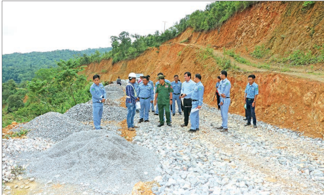
Union Minister Lt-Gen Ye Aung and officials inspect the construction of the road section in Kayah State. PHOTO: MNA
