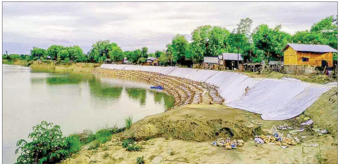
The almost completed embankment along the Mone creek is seen. PHOTO: YE WIN NAING (NYAUNG U)
