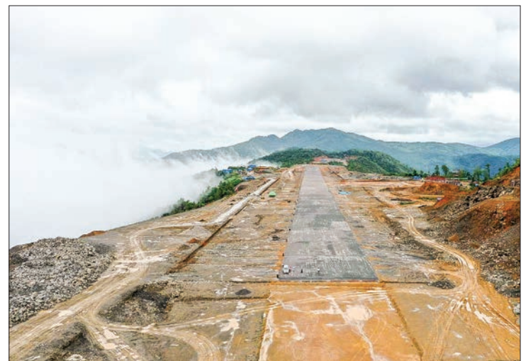
The view of Surbung Airport in Falam, Chin State which is under construction. PHOTO: YAMANYA
