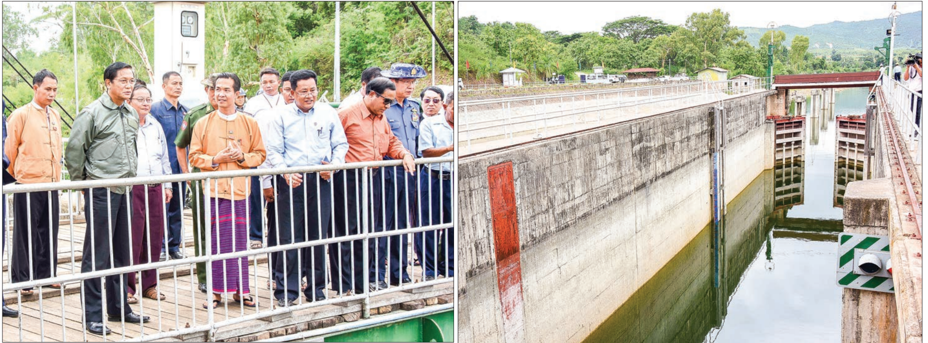
Vice President U Henry Van Thio observes the sluice gate which is also used for boat transport services, and the inflow of water into Moebyae Dam in Kayah State. PHOTO: MNA
