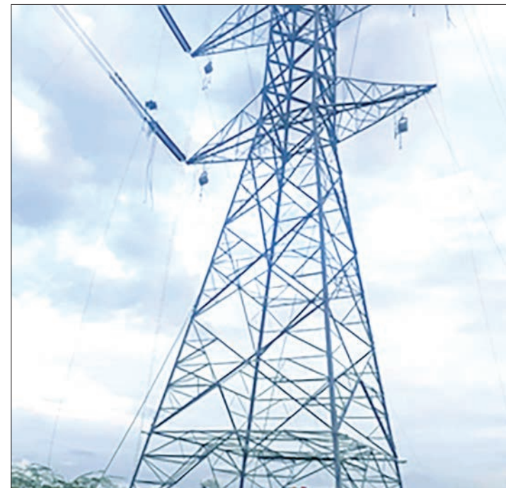
The 500 KVA transmission tower in Pyawbwe Township from which four Chinese people fell off. PHOTO: MPF
