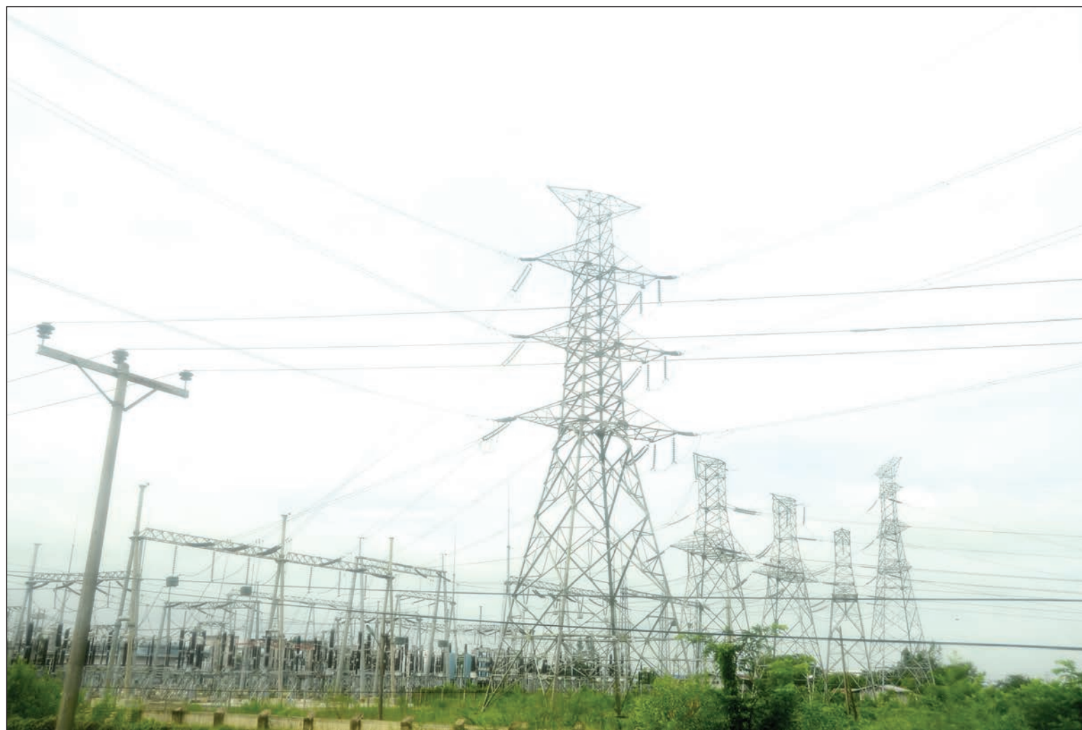
An electricity substation. PHOTO: PHOE KHWAR
