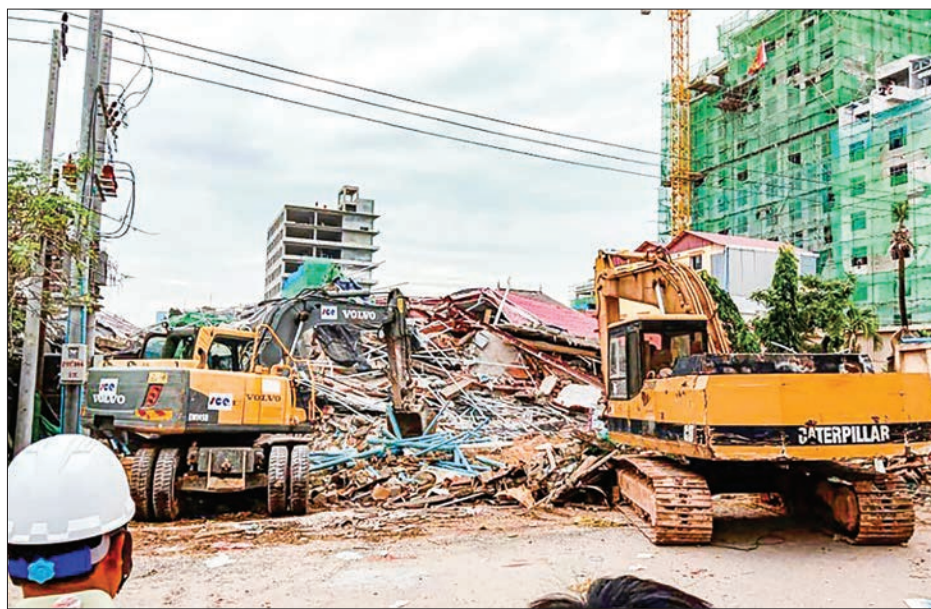
Dozens are feared buried in a building collapse in the Cambodian beachtown of Sihanoukville. PHOTO: AFP
