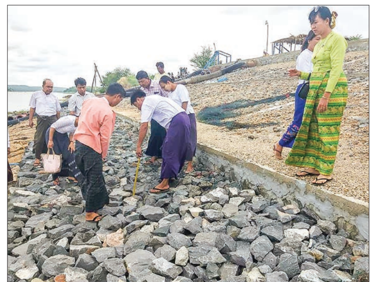
Officials check the construction of embankment along the Chindwin riverbank in Budalin Township. PHOTO: TOWNSHIP IPRD
