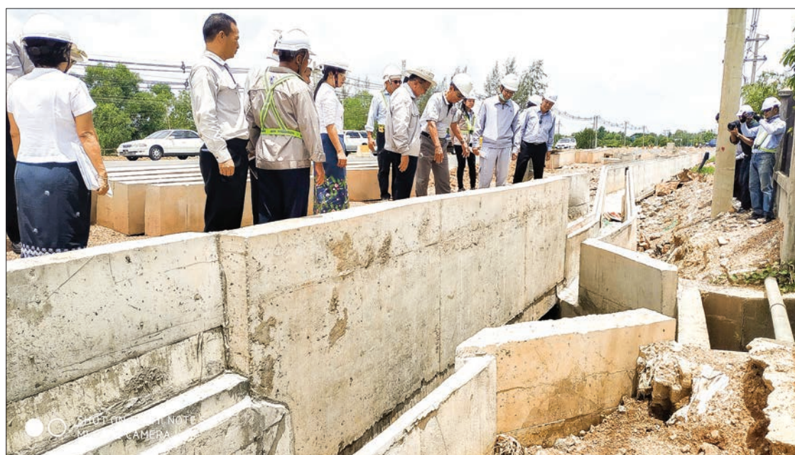
Union Minister U Han Zaw visits a bridge construction site in Yangon yesterday. PHOTO: MNA
