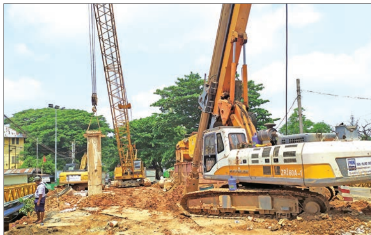
A view of construction work in progress on the flyover along Yangon Circular Railway. PHOTO: MYINT MAUNG SOE
