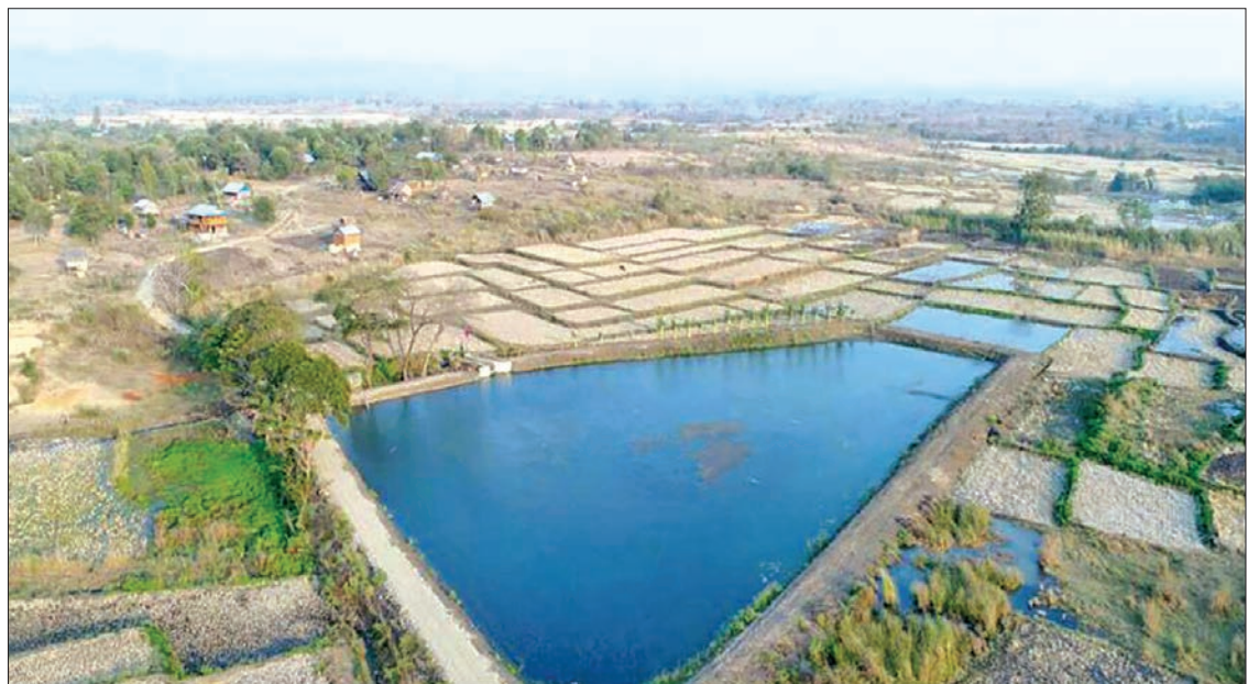
A reservoir near Wintgabar and Kyaung Gon villages in Ngaphe Township, Magway Region, undergoing renovation.
