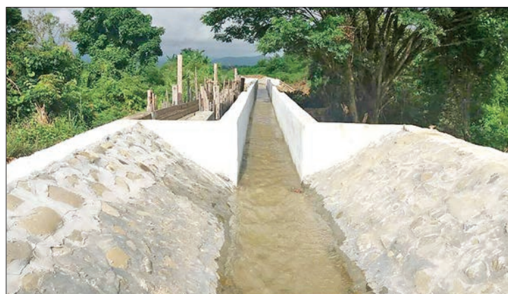
Ohk Poe Creek near Nham Khar village in Gangaw Township, Magway Region, undergoing reinforcing and renovations.
