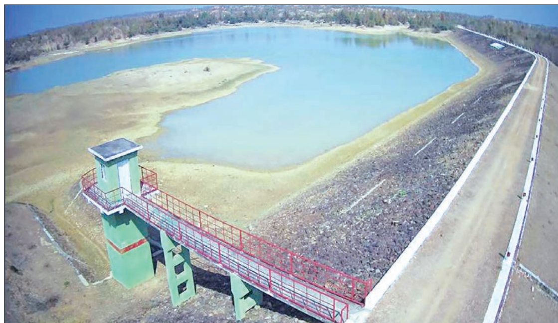
Nga Chin dam near Nga Chin village in Seikpyu Township under renovation.
