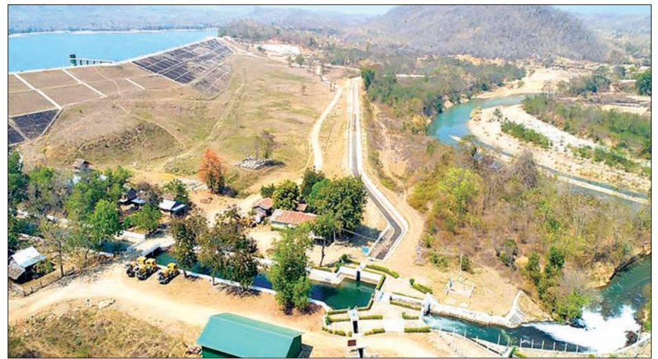
Rock lining underway along the embankment wall of Mahn reservoir in PinU Village, Ngaphe Township.
