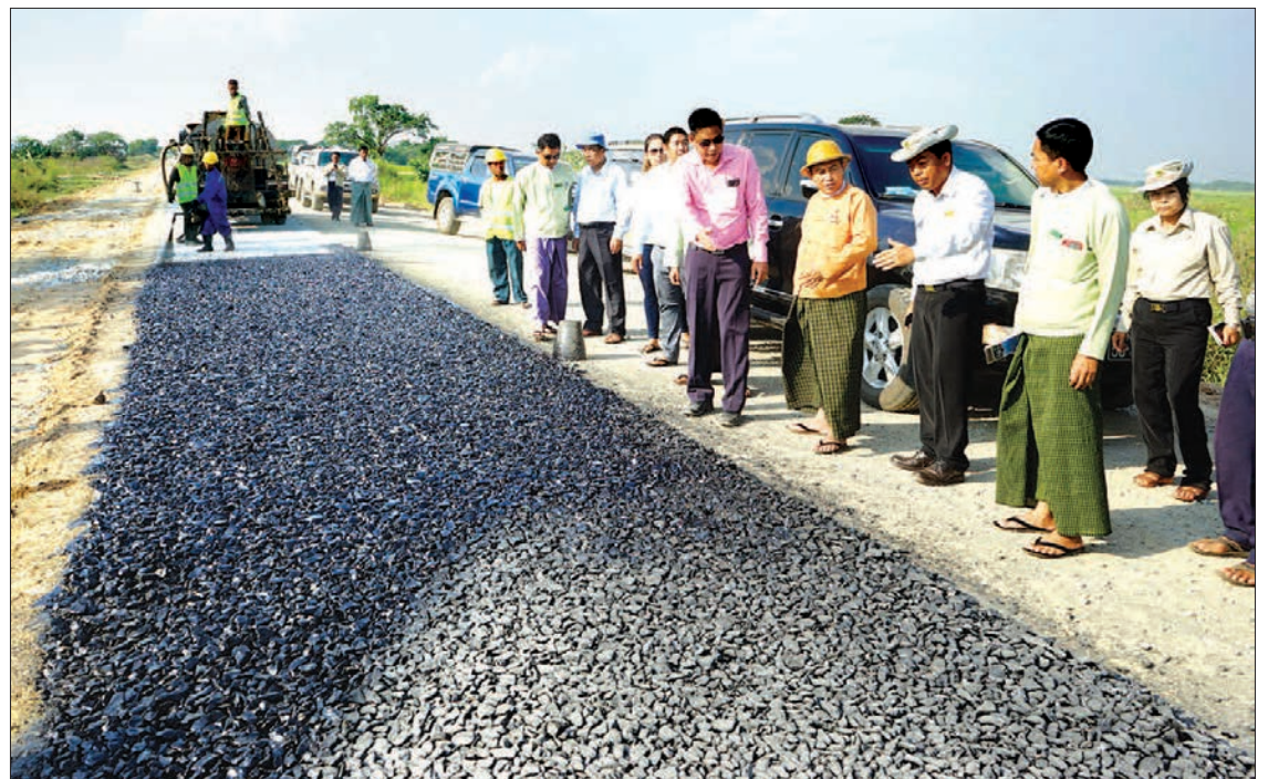
Bago Region Chief Minister U Win Thein, Hluttaw Representatives and departmental officials inspect the upgrading of the Daik U- Sittaung Road on 24 November, 2018. PHOTO: MNA
