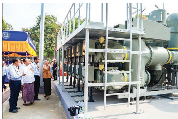
Union Minister U Win Khaing inspects the new Hline University GIS substation implementation. PHOTO: MNA
