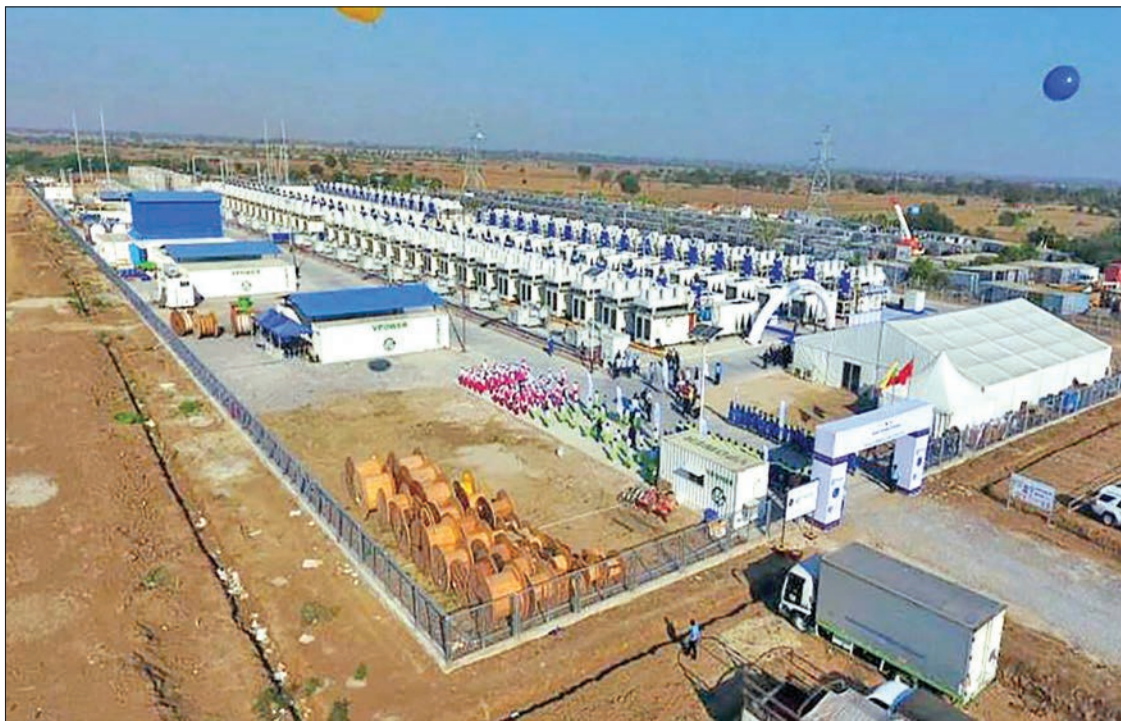
The newly opened 99-megawatt gas-fired station in Myingyan. The station will generate 90 megawatts in summer and 45 megawatts in the rainy season. PHOTO: MNA
