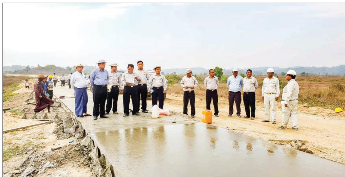
Deputy Minister U Kyaw Lin and officials inspect Angue Maw-Maungtaw road construction site in Maungtaw yesterday. PHOTO:MNA
