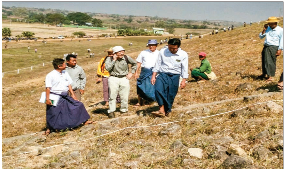
Local and foreign experts are inspecting a crack at the earthen embankment of the Taungnawin Dam in Paukkaung Township. PHOTO: NAY LIN (MNA)
