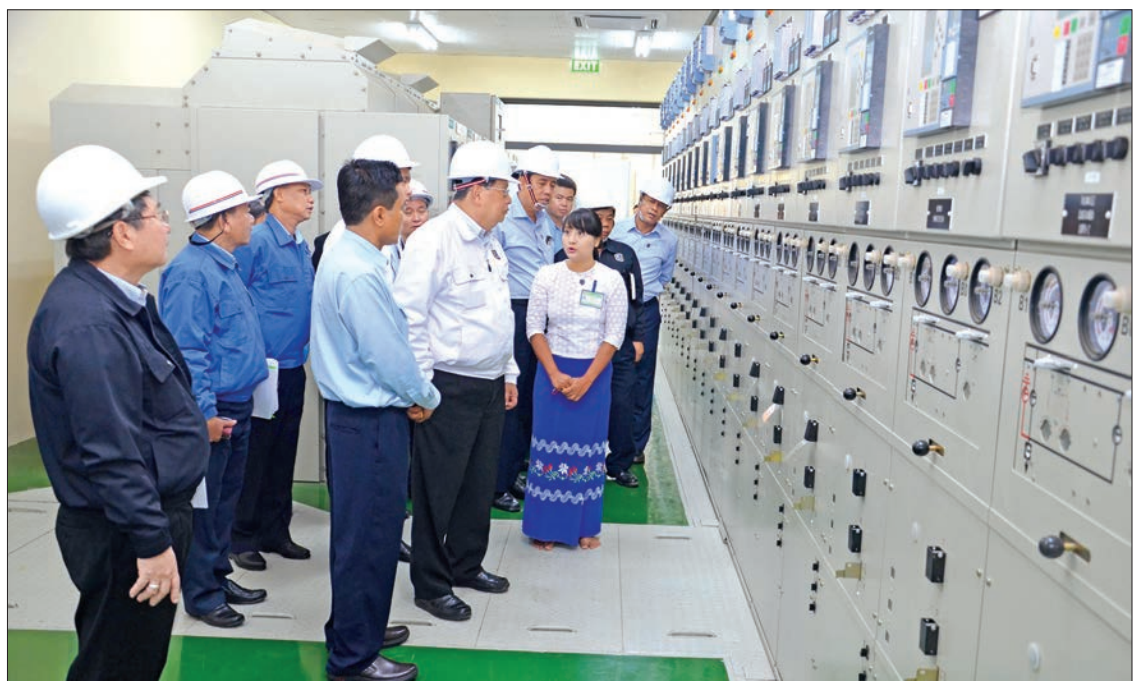
Union Minister U Win Khaing inspects a power plant during his tour of inspection in Yangon yesterday. PHOTO: MNA
